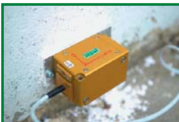
Vibration sensor on the wall
